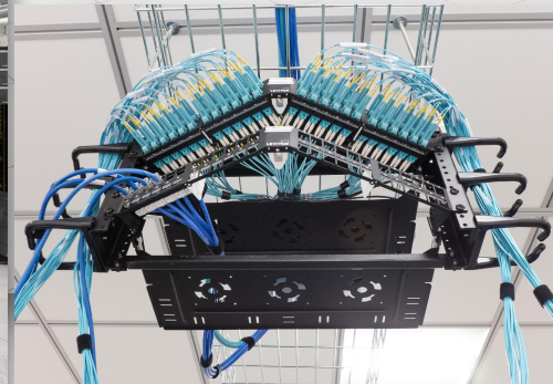
Typical overhead mini-rack serving fiber & copper connectivity
