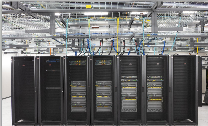
B725 Central Network Equipment Fully Deployed
