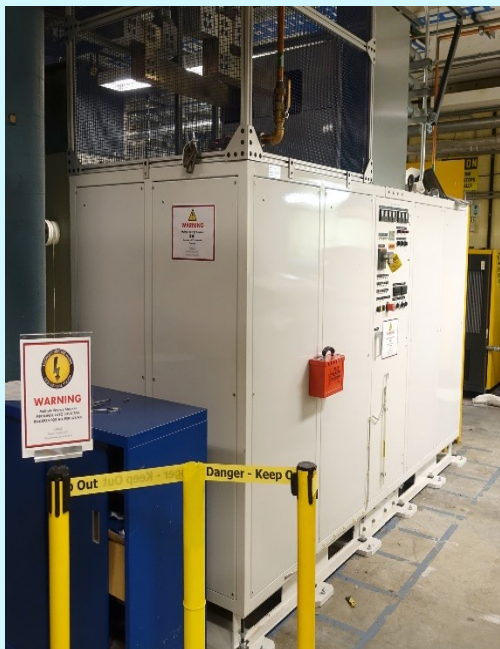
25kA Power Supply
